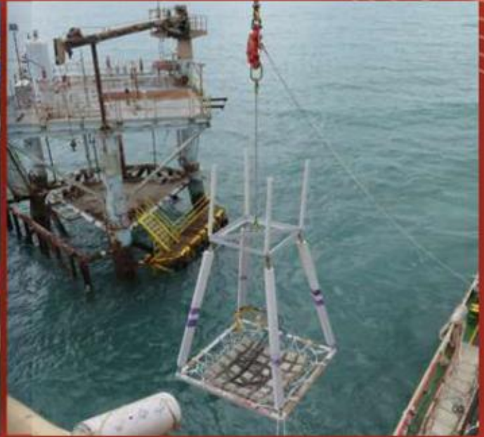
CP ANODE POD DEPLOYMENT PROCESS
